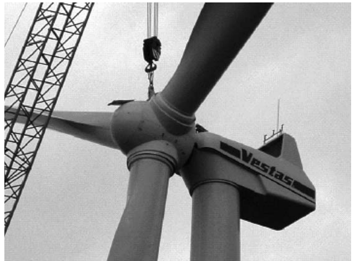
A 1.65 MW wind turbine. The blades are 40 m long and the hub is 80 m above ground
